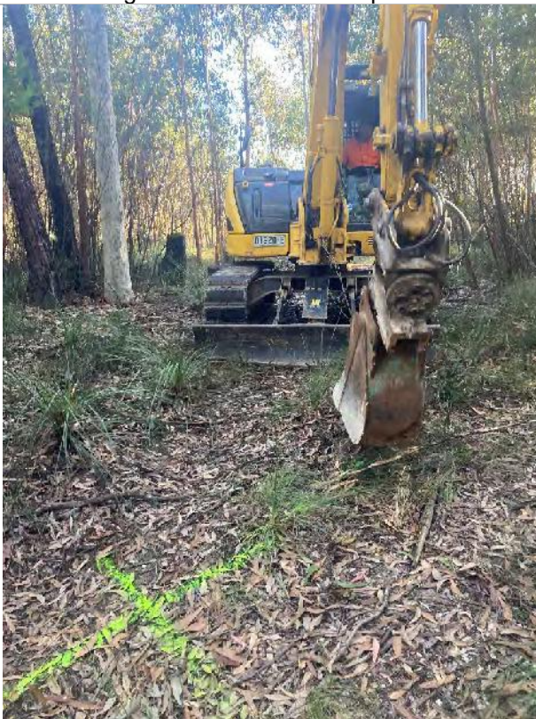
Photo 7: Sumitomo 8-tonne excavator used for test pit excavation in the Phase 2 development area.
