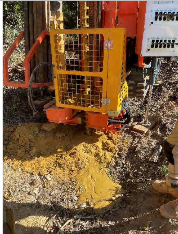
Photo 4: Groundwater encountered in the Phase 1 development area at BH12.
